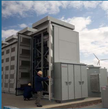
Xcell's 1MW / 6hr Sodium-Sulfur Facility Luverne, Minn. Complementing 11 MW Wind
